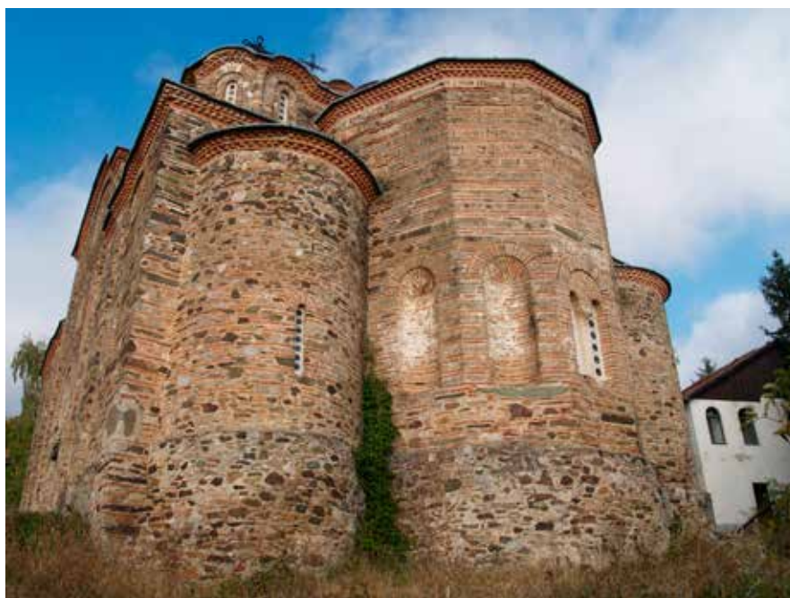
Fig. 8. General view from the east side: the apse and upper structure of the church (© Jasmina S. Ćirić)
